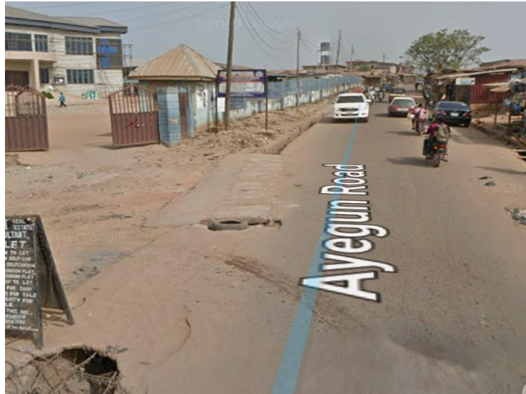
Plate II. Fanawole Junction, Ayequn Road, Apete, showing pavement deterioration along the study corridor.
