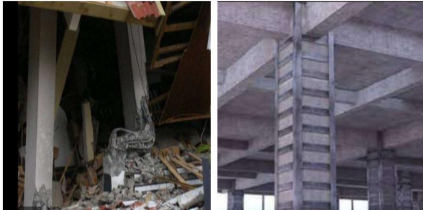
Fig.1. Earthquake damage and application of reinforcement to columns
